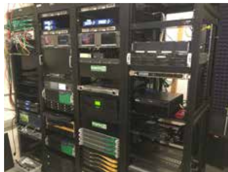
New Master Control Servers
